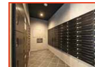
Installation of delivery boxes (Gran Casa Saitama Shin-toshin)
